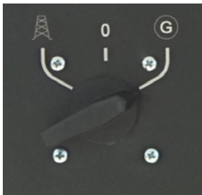
Main/generator selector switch
